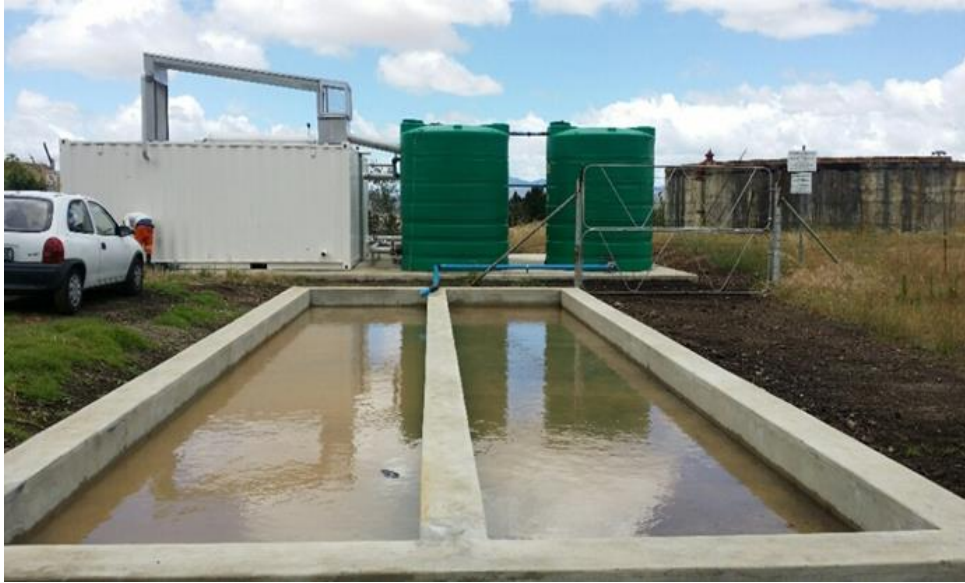
Hot Water Purifying Package Plant – Caledon
