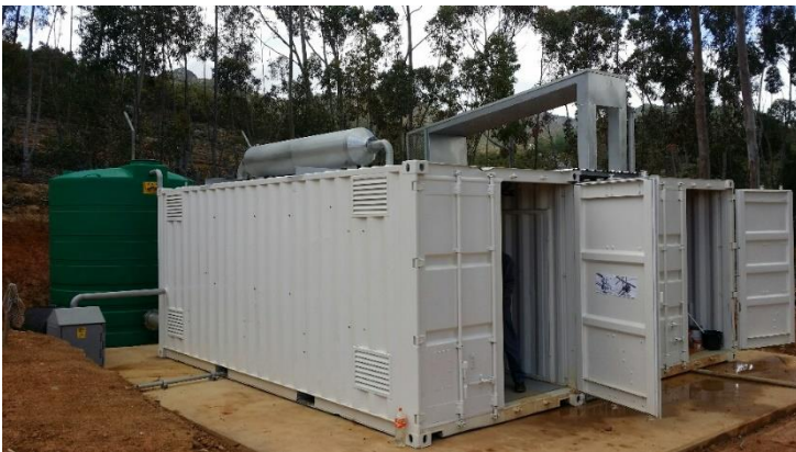
Package Plant at 4MI Reservoir – Caledon
